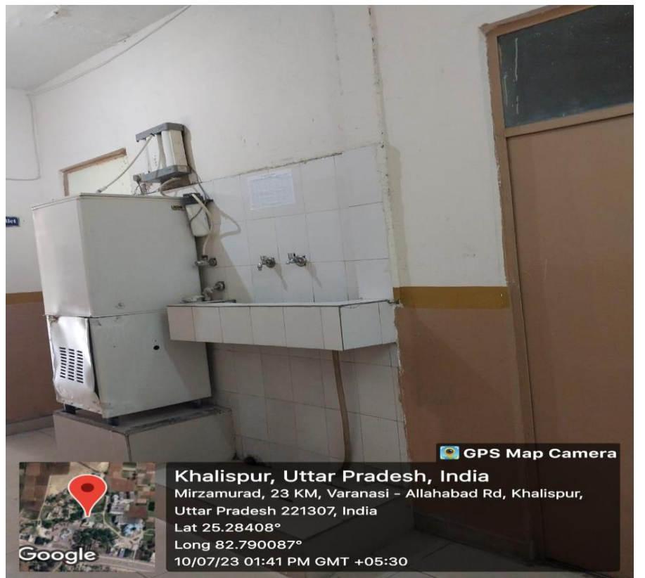
Water cooler with purifier (Second floor)
