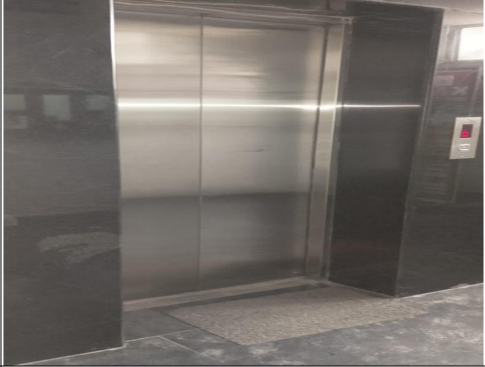
Lift in CRC Building
